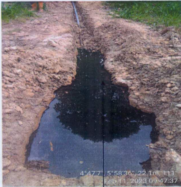
SPILL POINT BEFORE EXCAVATION
